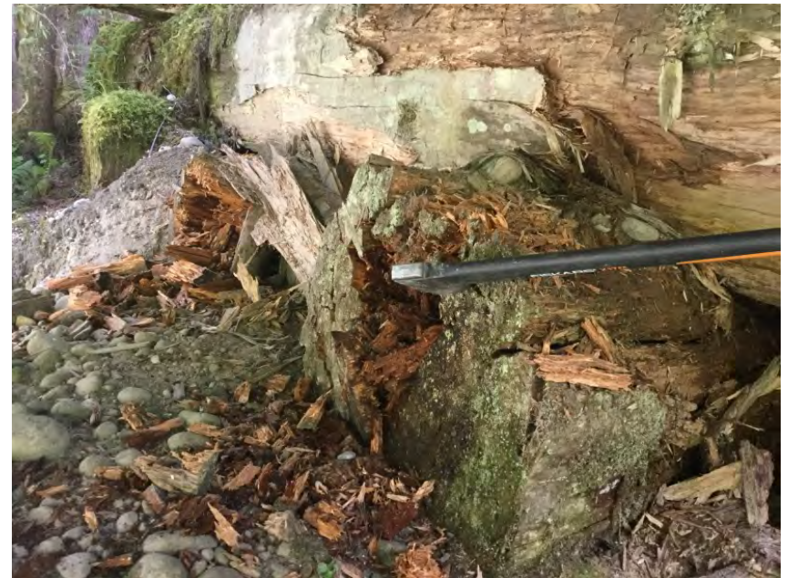
3 of 5 Mud sills on right bank rotten, only upstream and downstream still competent with 100mm sap rot noted
