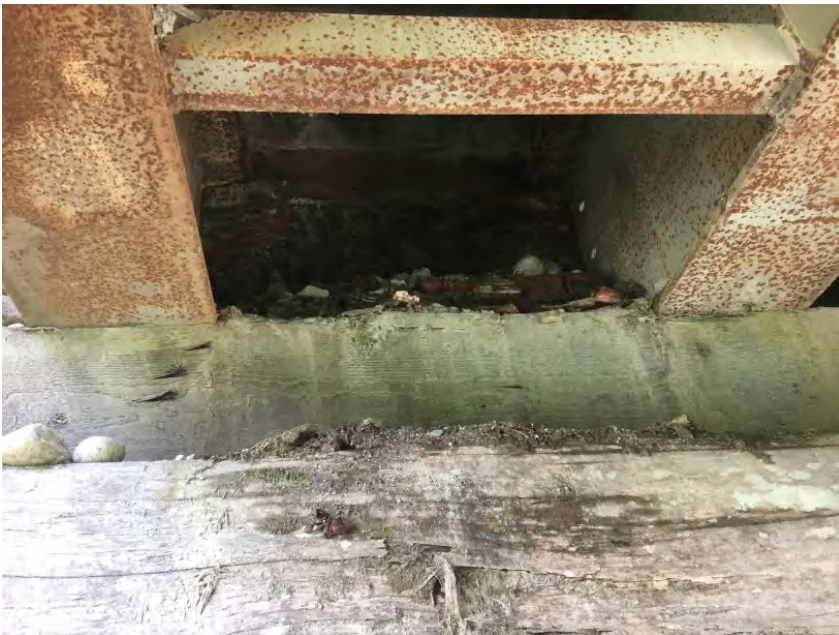
Left bank ballast wall non existent in locations
