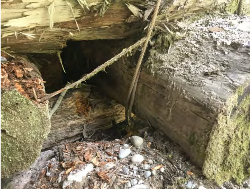
Upstream mud sill competent but bearing on rotten log in fill
